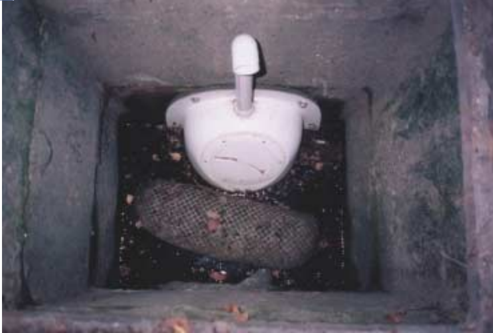
12 F SNOUT and Oil Boom in a 2' x 2' inlet structure with an 8" clay outlet pipe with 18" of sump in the structure below pipe invert. This unit functions as an inlet oil-water separator reducing oil, grease, and floatables that are discharged to a pond.
