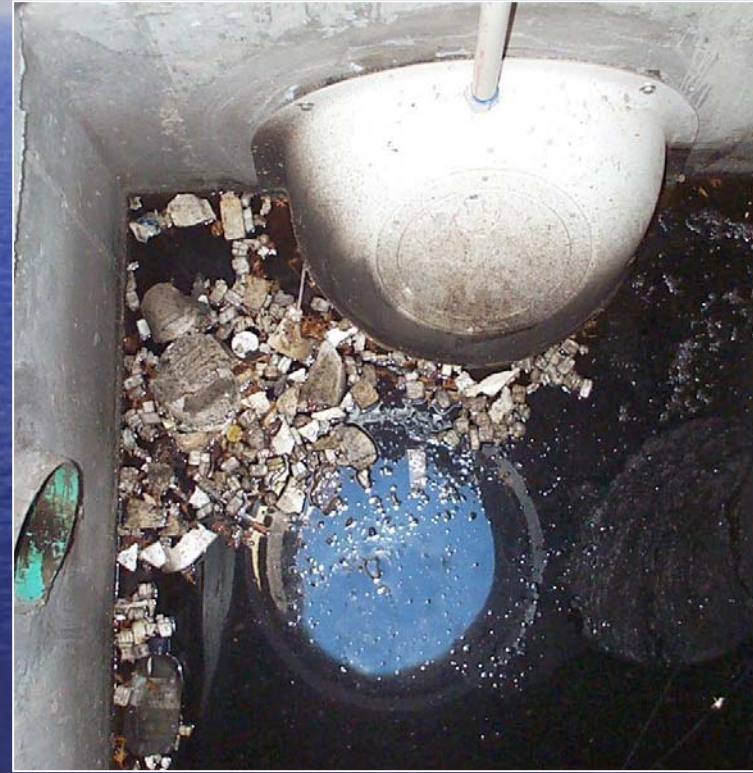
Structure with SNOUT stopping oil and debris from upstream. Site is in West Valley City, Utah. Installation was featured in 2004 Stormwater Magazine Article.
