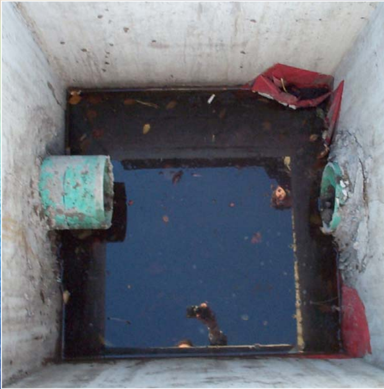
Inlet shown with no SNOUT that flows into structure with SNOUT. Water clear, no oil, little trash.
